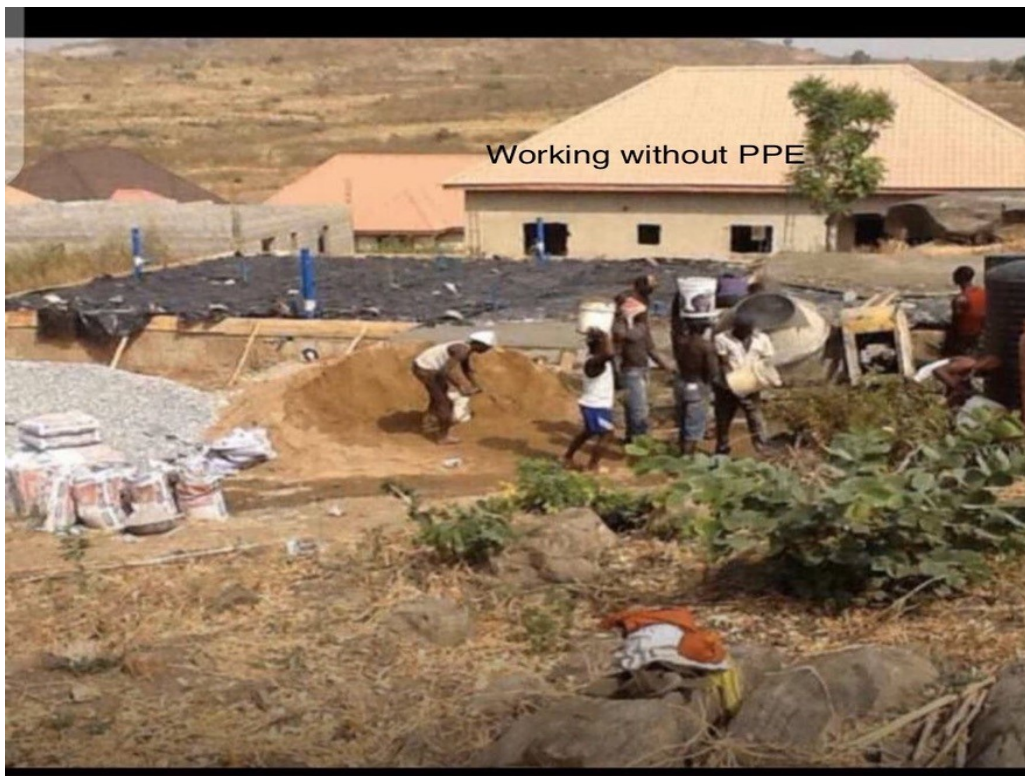
Figure 3: Workers without PPE on a construction site in Nigeria (Picture submitted by site supervisor)
