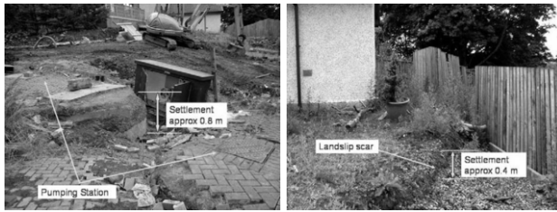
Figure 2. Magnitude of settlement around the pumping station and in the garden of the adjacent house .
