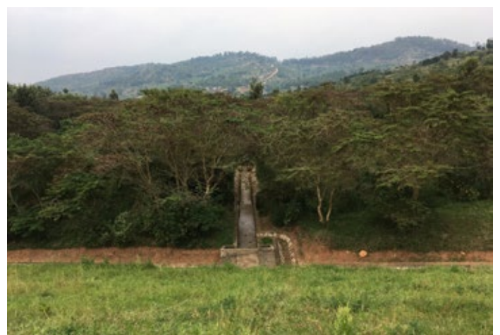
Figures 7 and 8: Local dam in the Huye District, which provides water to the cooperative's rice paddies downstream. Side view (top) and downstream view (bottom).
