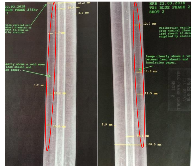
(a) Front images (b) Rear images – the red ellipse shows the area of oil leakage
