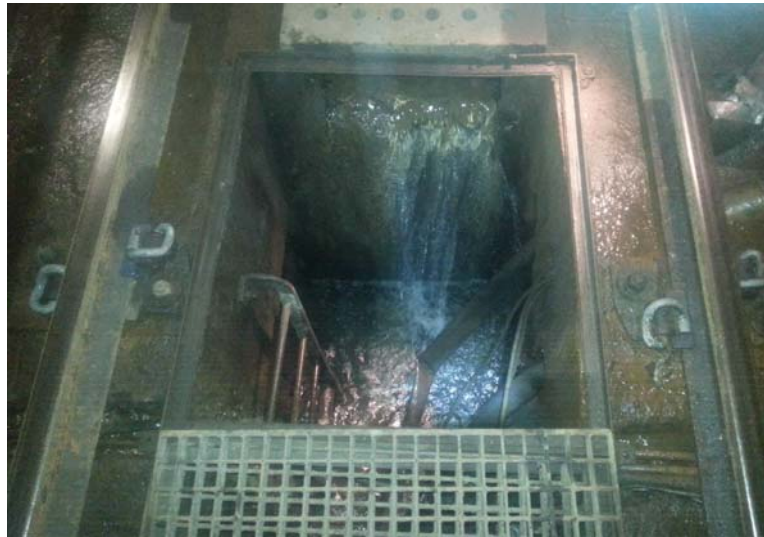
Figure 2: Sump located between the rail tracks in the Glasgow Subway system
