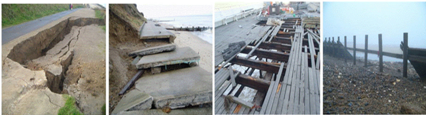
Figure 2: Post storm-surge damage to various NNDC coastal assets.
