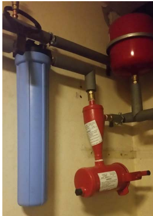
Figure 9: The water filter at the plant room
